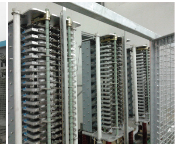
Indoor thyristor valve
